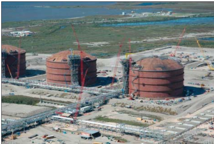
Construction progresses on tanks for Cheniere Energy's Sabine Pass LNG terminal. Each tank is capable of storing 160,000 cu m of LNG. The terminal will be completed in second-quarter 2008. Photo from Cheniere.
